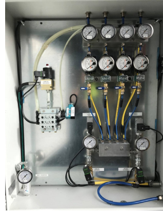
+ Four Edger Saw Lube System
